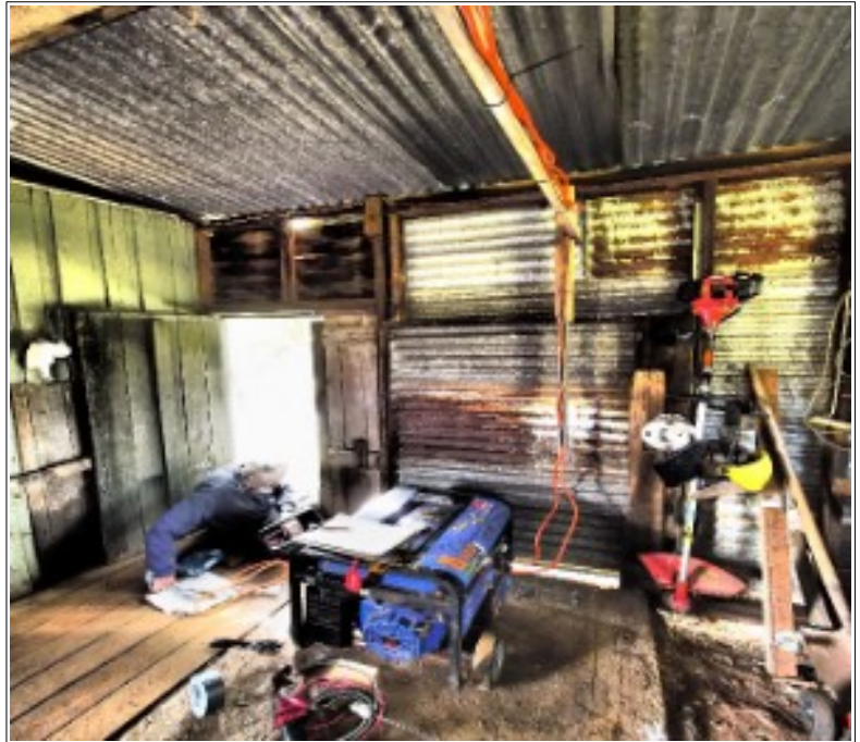
The generator in a new position in the machinery shed
